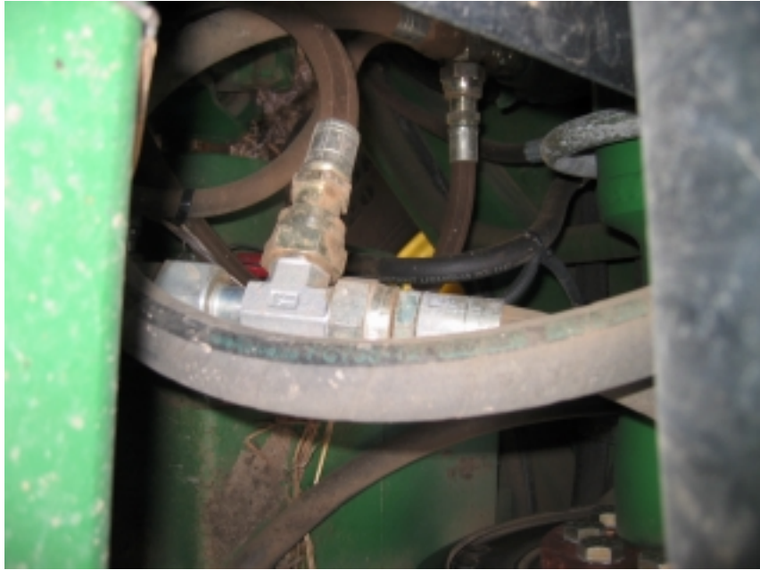
Figure - Another Showing "Tee's" into hoses for pressure and tank
