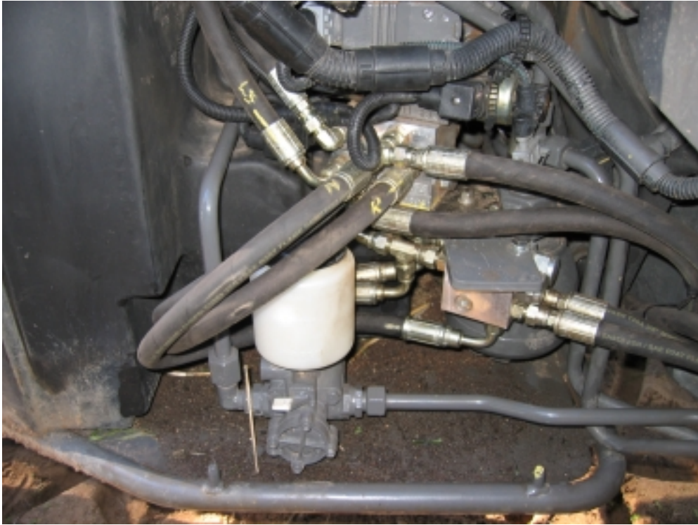
Figure- Steering and lockout valve in behind tractor hydraulics cover. RHS of tractor
