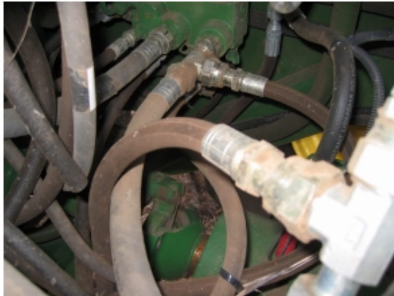
Figure - Showing "Tee's" into hoses for pressure and tank
